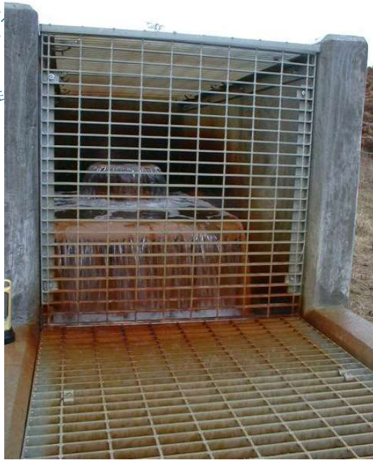
Groundwater is pumped to the surface & aerated
