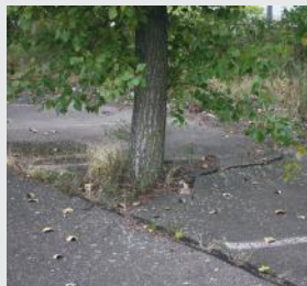
Some bore holes were drilled directly into asphalt paving areas. Poplar cuttings were not affected.
